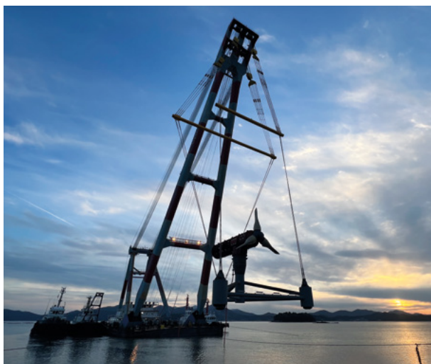
Tidal turbine installed at the Uldolmok tidal energy test site. © KIOST
