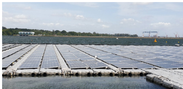
Figure 10: 1.5 MWp floating solar PV system at Lower Seletar Reservoir
