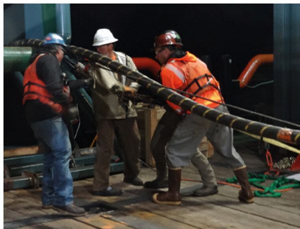
Teams work offshore to finish laying subsea cables for the PacWave South test site. © PacWave
